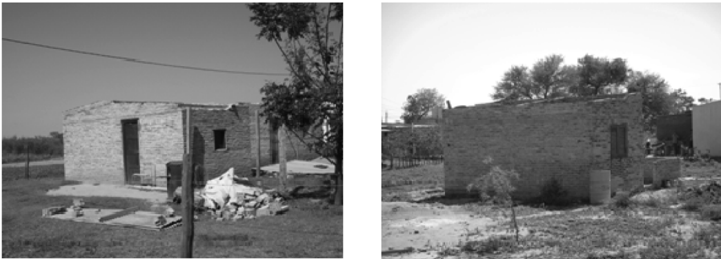
Fig. 9 These are examples of typical Class 2A structures. Both houses were unroofed during the storm described in section 3.5
