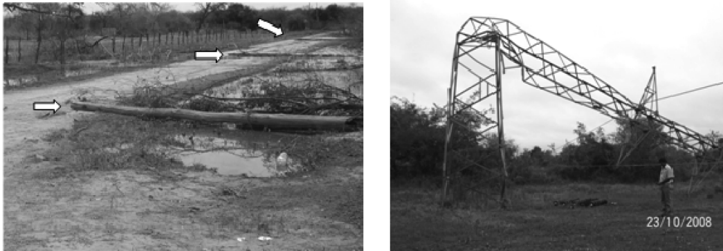
Fig. 11 Vulnerable electricity line poles. Left: Creosote-treated timber poles used in low-voltage lines; right: a 132-KV line supporting tower (photograph courtesy of Ing. Miguel Malarin)
