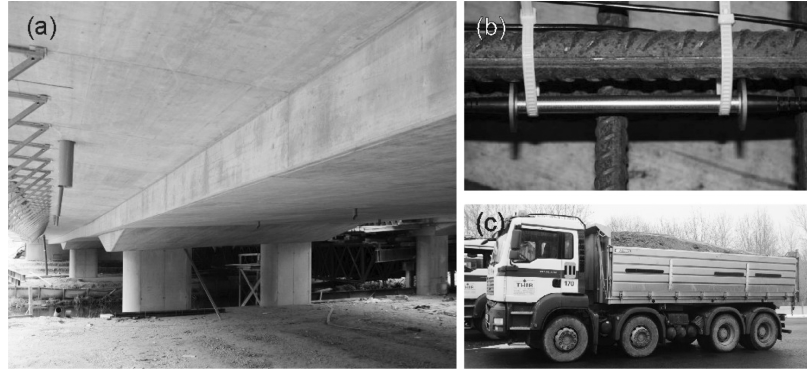
Fig. 3 Case study “Marktwasser Bridge S33.24”: (a) Side view - Picture taken from North - East, (b) typical installed fibre optical sensor and (c) vehicles for the proof loading campaign
