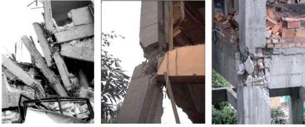
Fig. 1 Joint damageability and collapse of structures: from left to right: 1999 Izmit earthquake, Turkey, 1999 Chi-Chi earthquake (Taiwan), 1994 Northridge earthquake (USA) (Sharma 2013)
