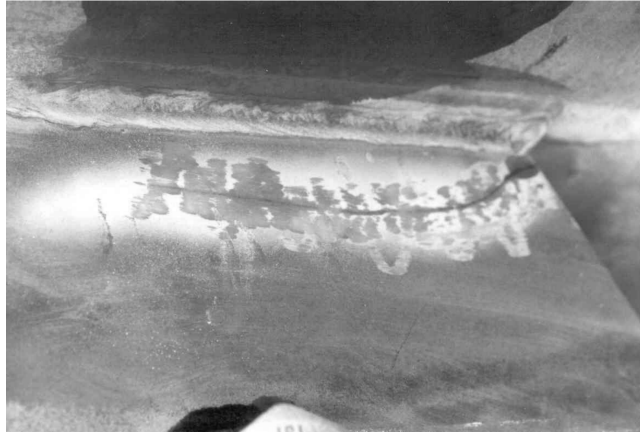
Fig. 11 Cracking in gusset due to LMAC
