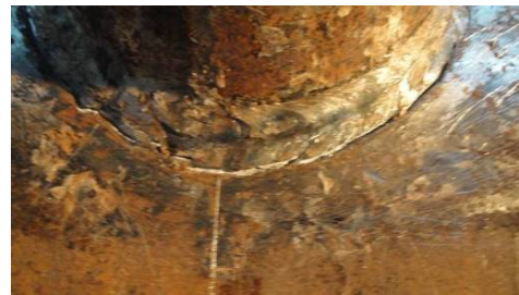
Fig. 6 View of crack along weld toe
