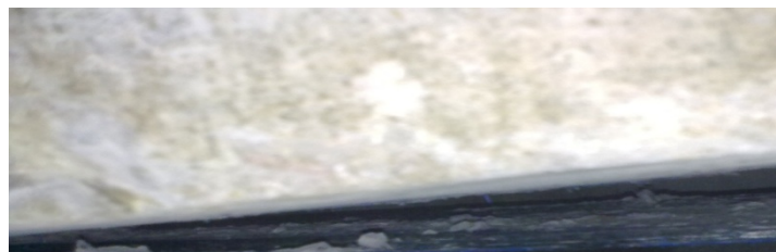
Fig. 11 Debonding of CFRP sheets in girders RDB1, RDB2, and RDB3
