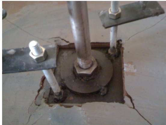
Fig. 11 Rigid steel footing resting on untreated soil
