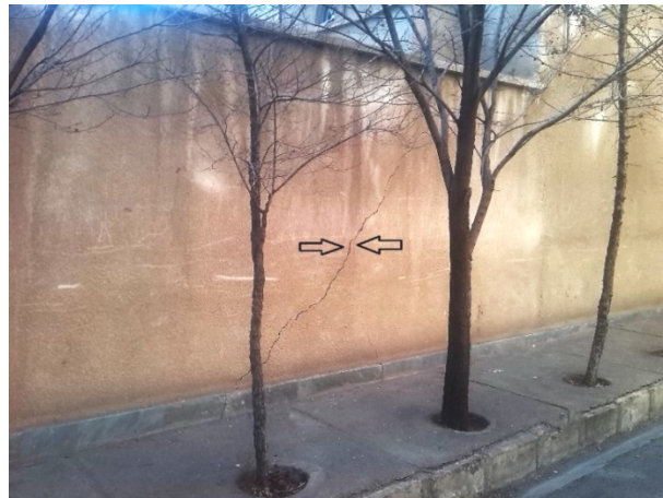
Fig. 2 Swelling in marls and creating crack on the walls
