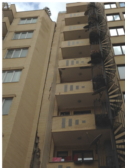
Fig. 4 Partial damage in building due to the differential settlement on marl layers
