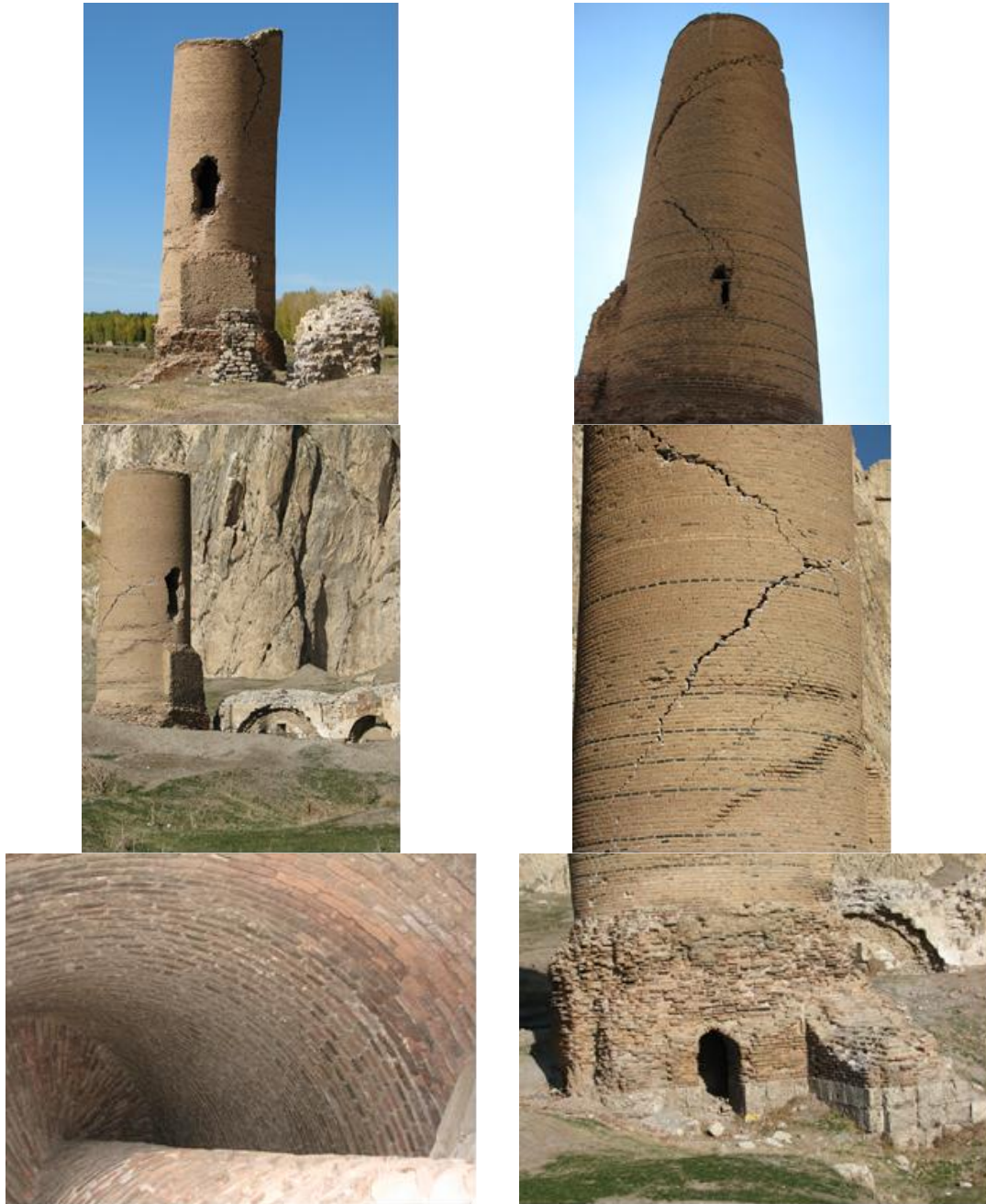
Fig. 6 The view of the deteriorations and damages on Ulu Mosque Minaret
