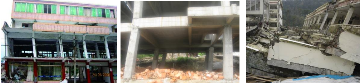
Fig. 2 Photos of the seismic damage of RC frame in Wenchuan Earthquake Region
